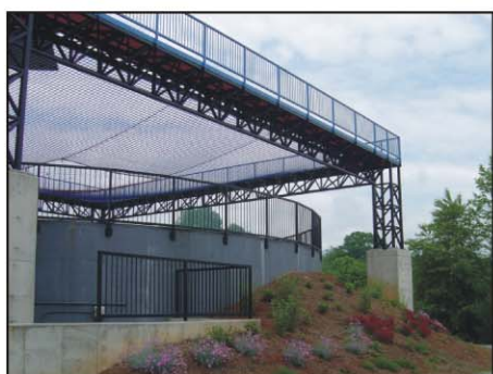
A view of the tunnel outlet and the flying net and walkway above it.
